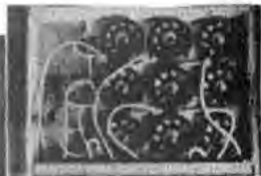
Switchboard with back removed to show rheostats, main switch, and color switches.
