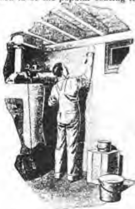
FIG. 40.—One coat of cold water paint makes an excellent and inexpensive basement paper.
