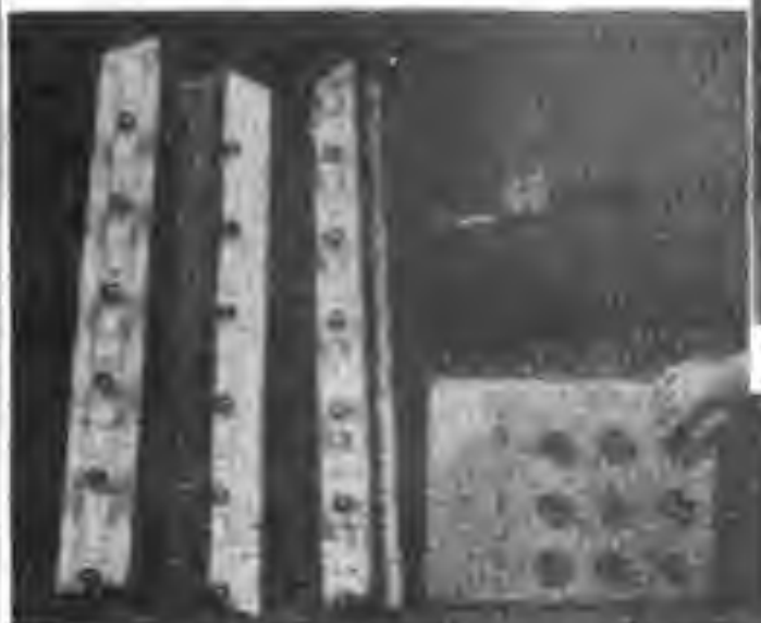
Footlights, border lights, flood light, and switchboard with four switches, rheostat knobs, and receptacles in edge.
